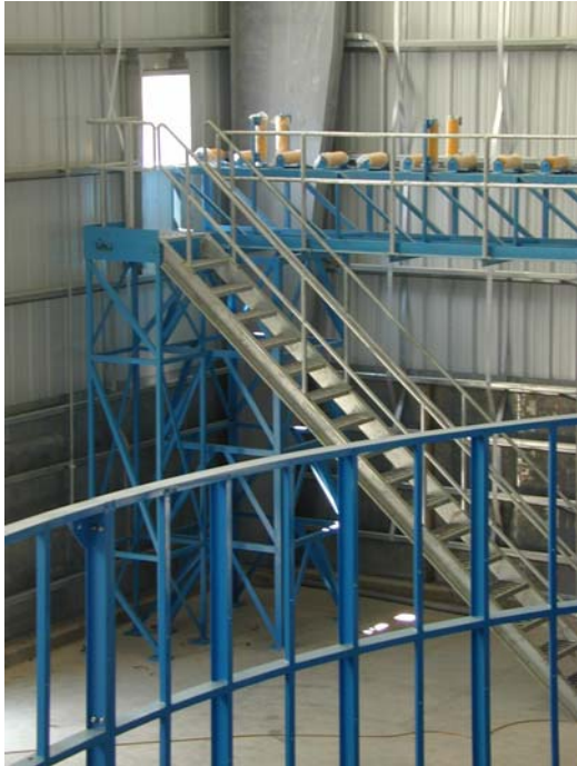
Typical product gantry with support roller track and access stairway.
